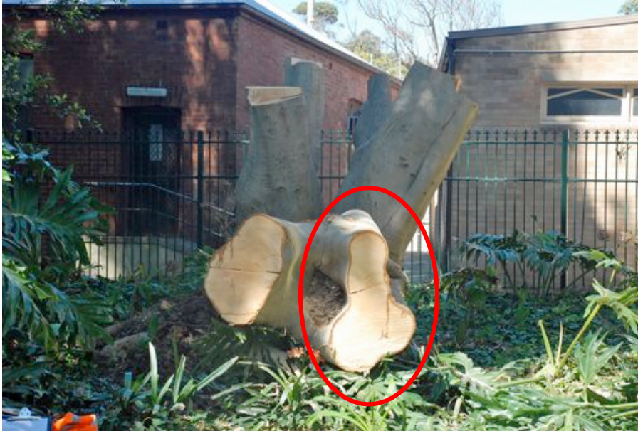
Photograph C. I-beam shape of failed stem, September 2008.
